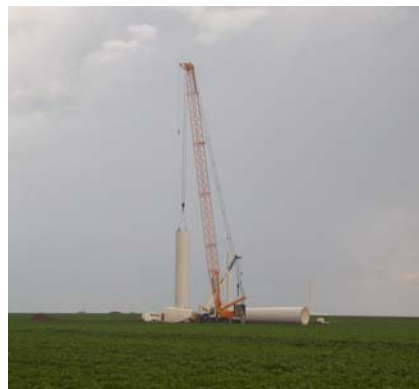
Heavy-duty cranes hoist components of Mitsubishi 1.0 MW turbines into place in the fertile cotton fields of Nolan, Mitchell & Scurry counties in Airtricity's 209 MW Roscoe project.
