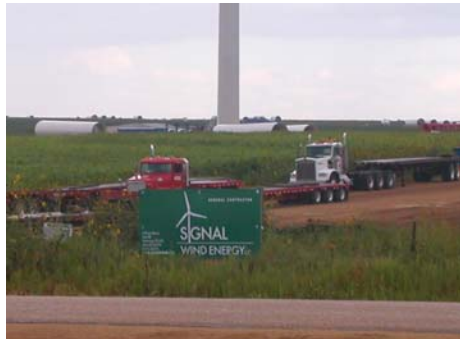
Vestas 3.0 MW turbines on 105-meter towers are now rising at the Snyder Wind Project.
